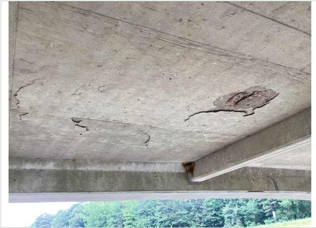
Span 1 bottom deck impending spalls and spall to steel
