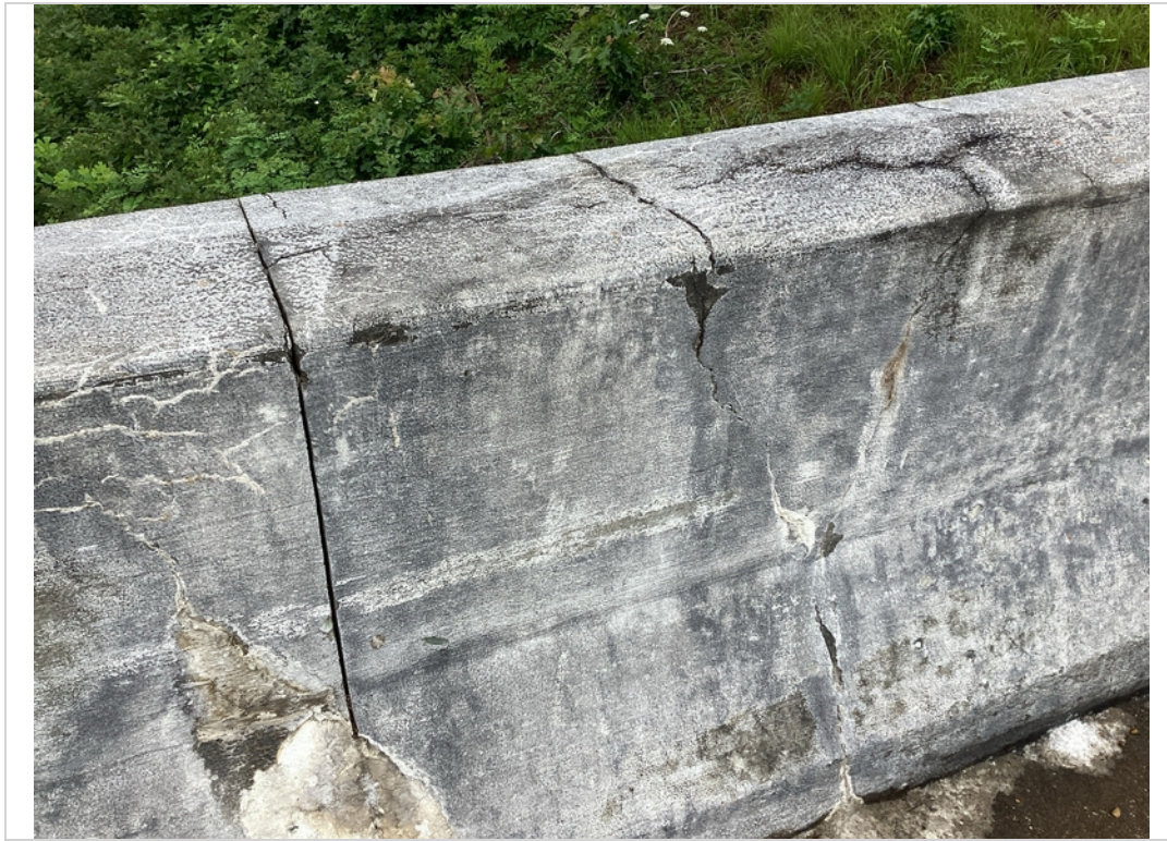
Span 1 parapet crack
