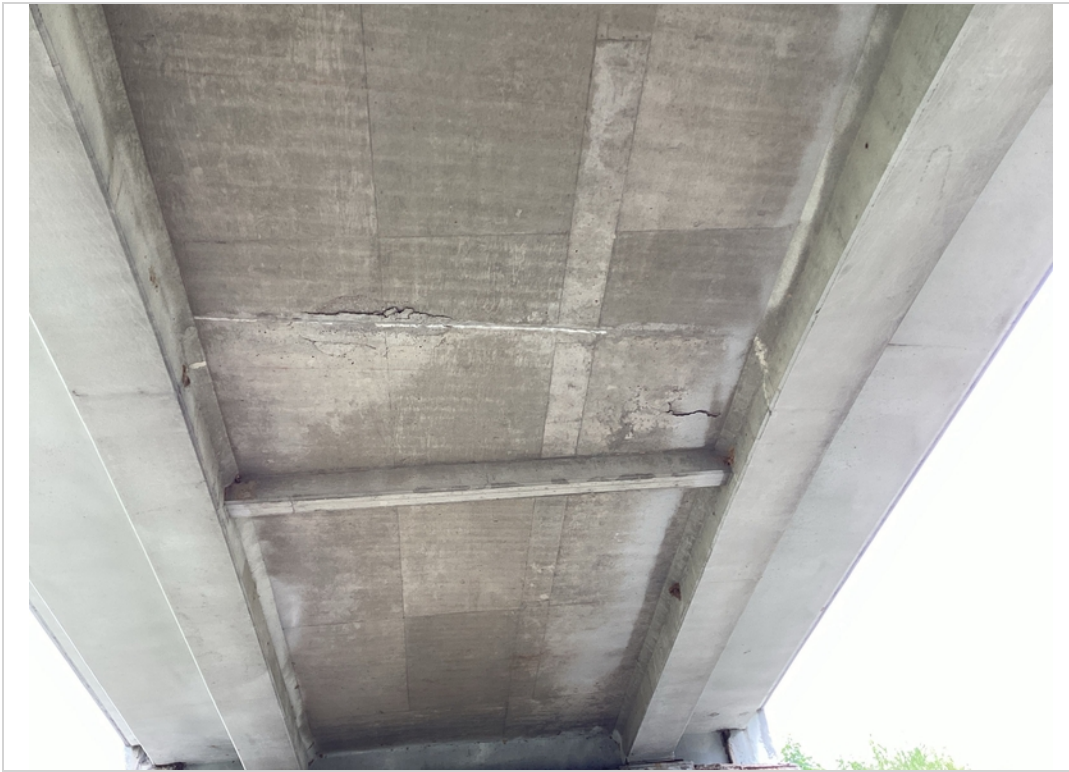
Impending spall on bottom deck of span #3
