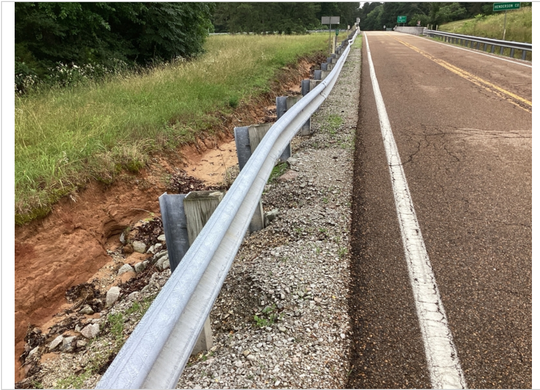
Approach 1 right guardrail damage
