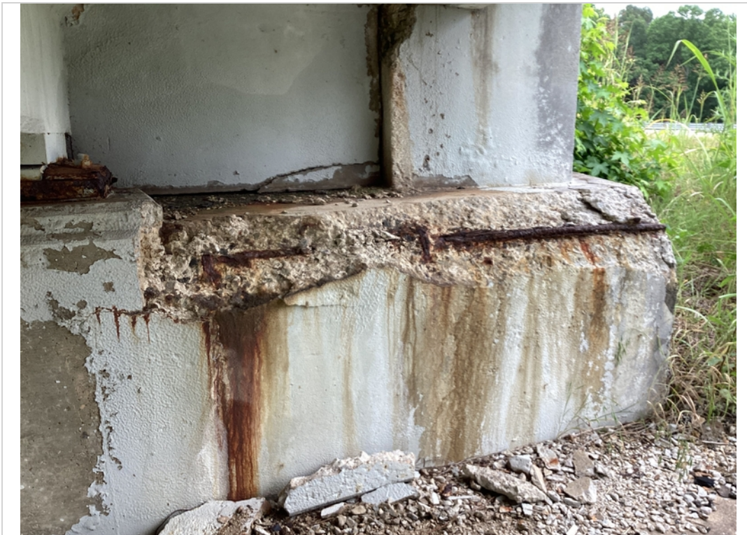
Spall steel abut 2
