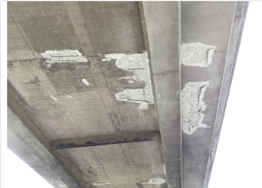
Span 2 bottom deck spall to steel
