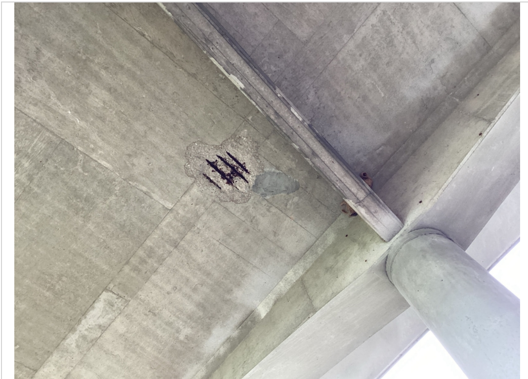
Spall to steel on bottom deck of span #3
